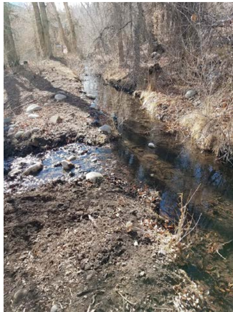
Figure 4. Example of Ditch Bank Breach
